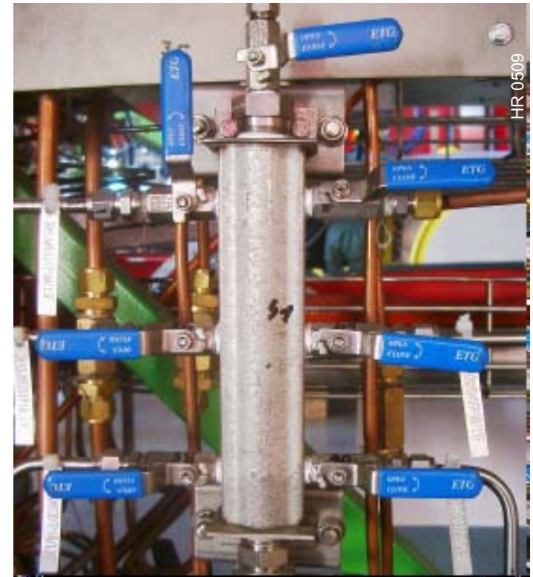
Cooling valves around a distributor.
