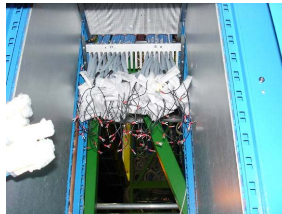
RPC sgn cables S11
