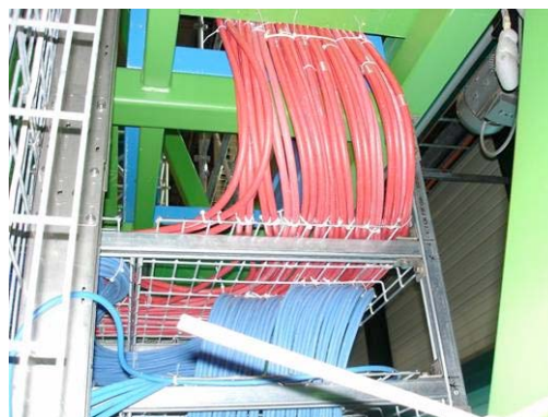
X3J22: HV DT cables
