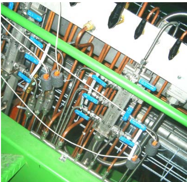
Distributor, with 4 sensors installed
