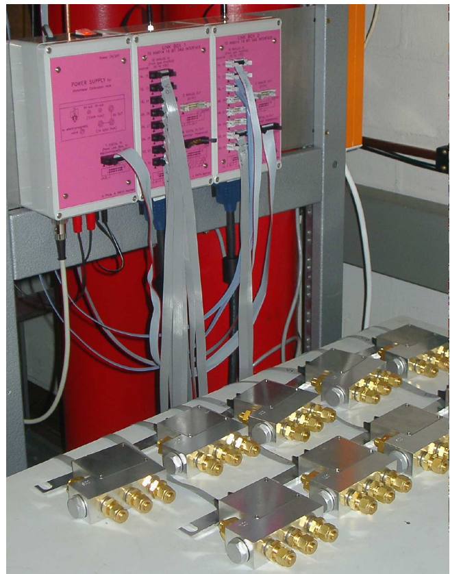
Calibration rack, side view: first 10 manifolds being connected, for simultaneous calibration (Dec. 2002).
